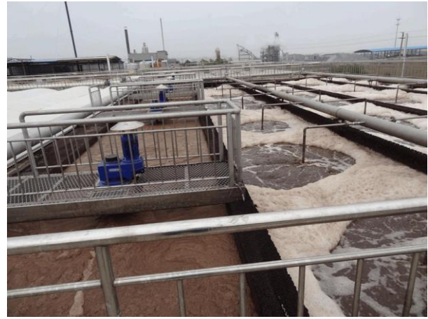
Photo 1: Pre-denitrification and aerobic biological treatment
