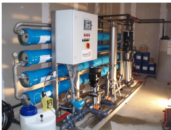
Picture: 1: Nanofiltration plant installed in France
